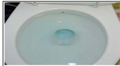
Figure 7 – Dye leaking into bowl
